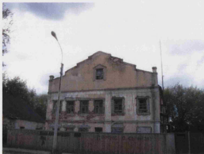
Figure 36 Derelict Building, Ivanovo City Centre, September 2006.
